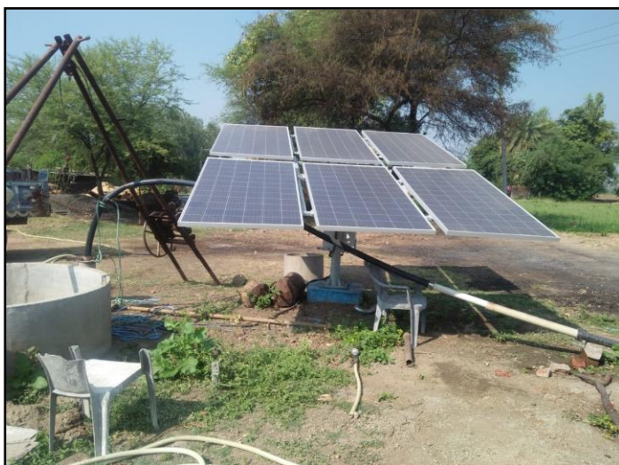
Solar pump Chainpura, Sehore District
